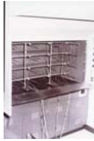
Photo 2 - Pitot-Static Tube Array for Fume Hood Face Velocity Sampling
